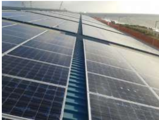
Solar panels on warehouse roofs
